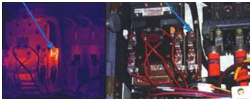
Figure 6.2.5. Overload connection problem. Note difference in IR image coloration between overload contacts.
