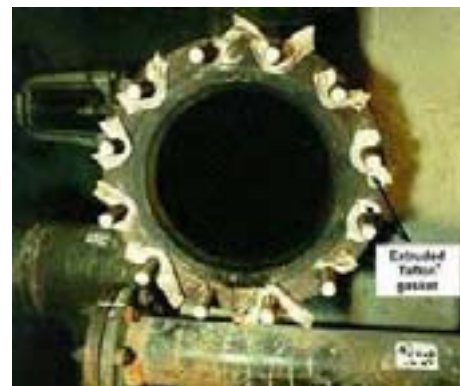
Figure 9.3.7. Failed gasket on blind flange.
