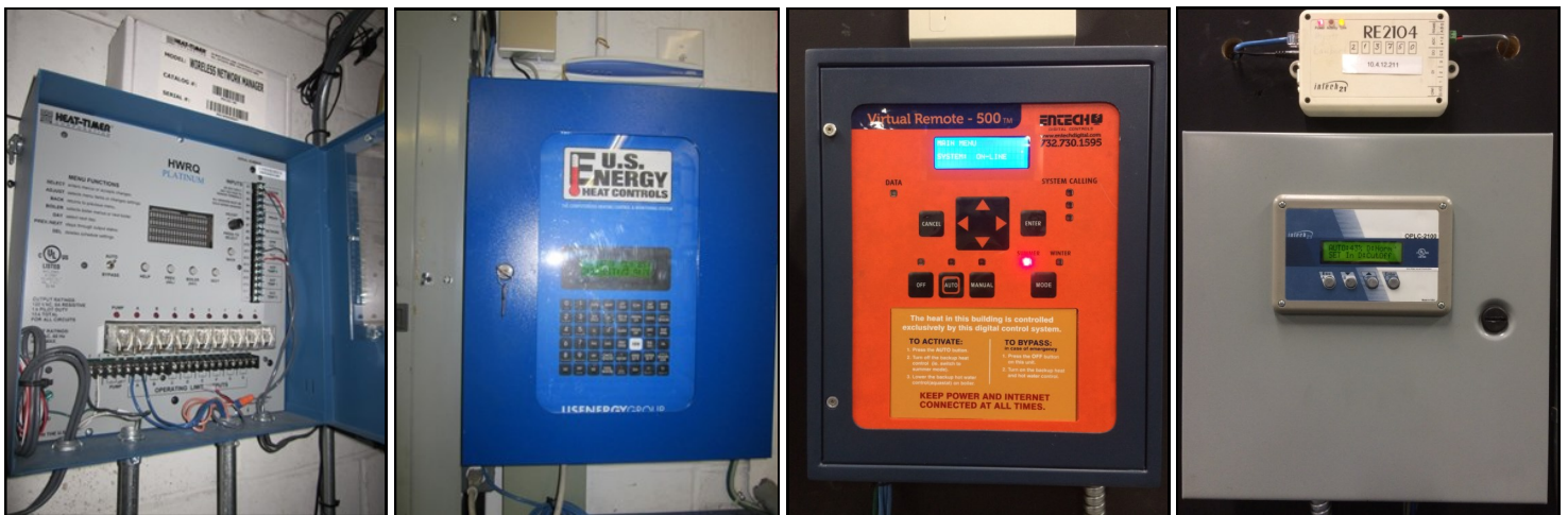
Figure 1: Central computers of Energy Management Systems installed in the field and manufactured (from left to right) by Heat-Timer, U.S. Energy, EnTech, and Intech 21. Photo credits: Far left and left by Taitem Engineering; right and far right by the Association for Energy Affordability.
